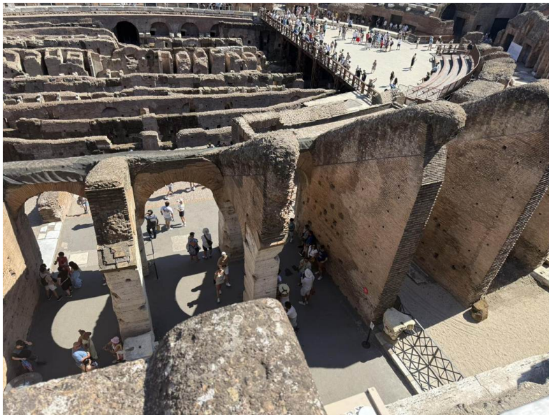
Inside: the radial walls and vaults that once carried the tiered seating (the cavea).
